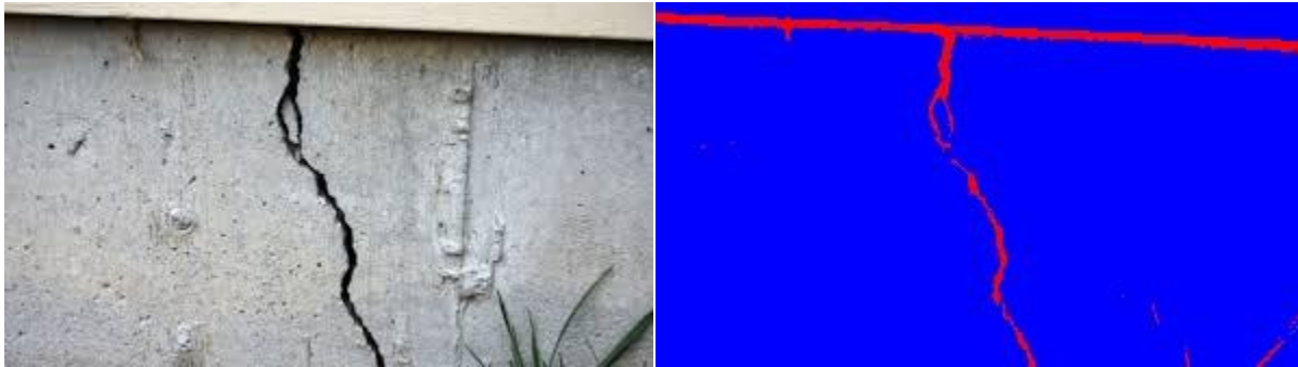
Figure 3: Data of cracks and segmented cracks
